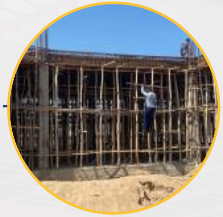
Amoud Foundation has begun construction of The Farah Egal Library which is the largest library in the region and will serve 1/2 million people in the region. It will also serve 5 schools and a technical school in the region.
